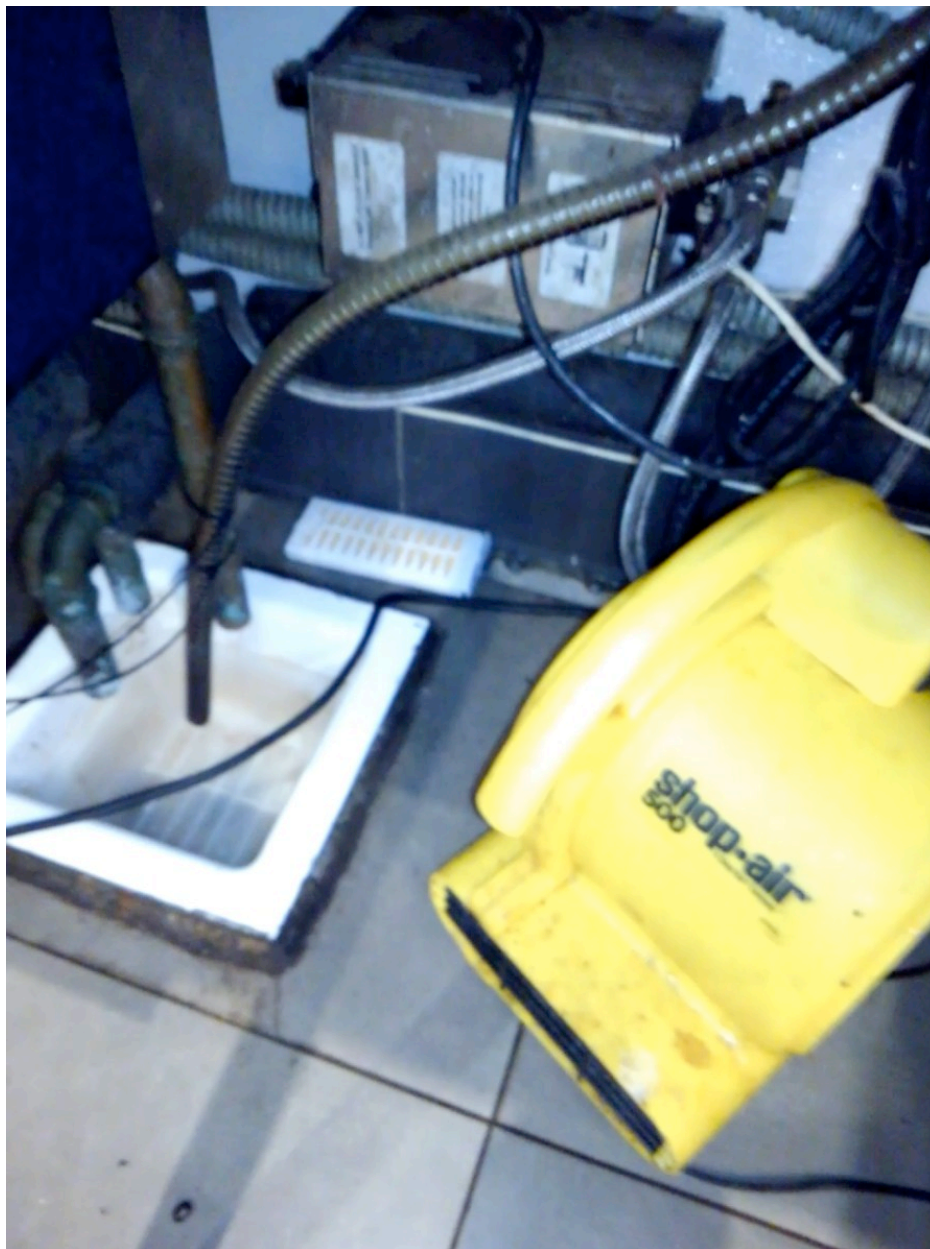
Port Authority, South Wing (March 1, 2017) DDVP No-Pest Strip Alongside Active Fan System, Circulating Vapors
