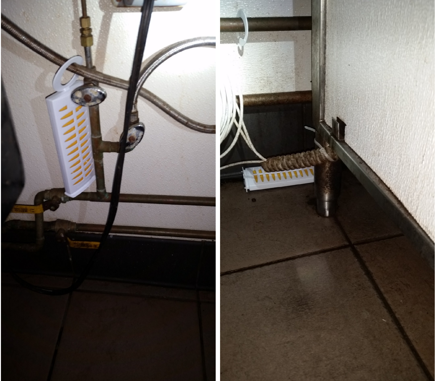
340 Madison Avenue (Oct. 14, 2015) DDVP No-Pest Strips Hidden Below Sinks
